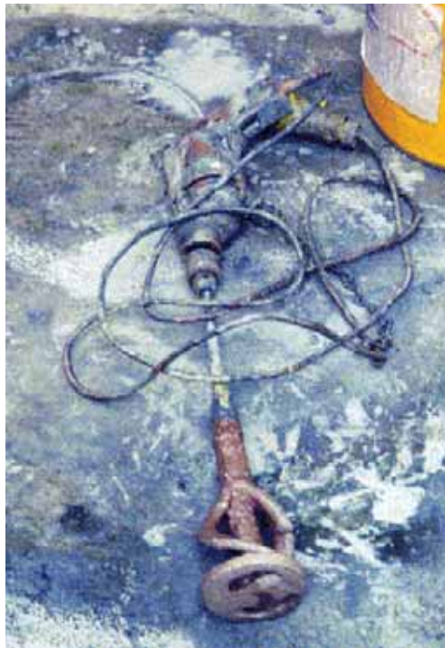
3. Required mixing equipment
